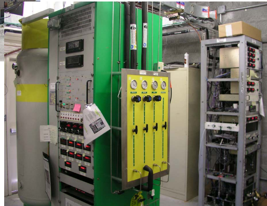
IFR gas mixing racks
