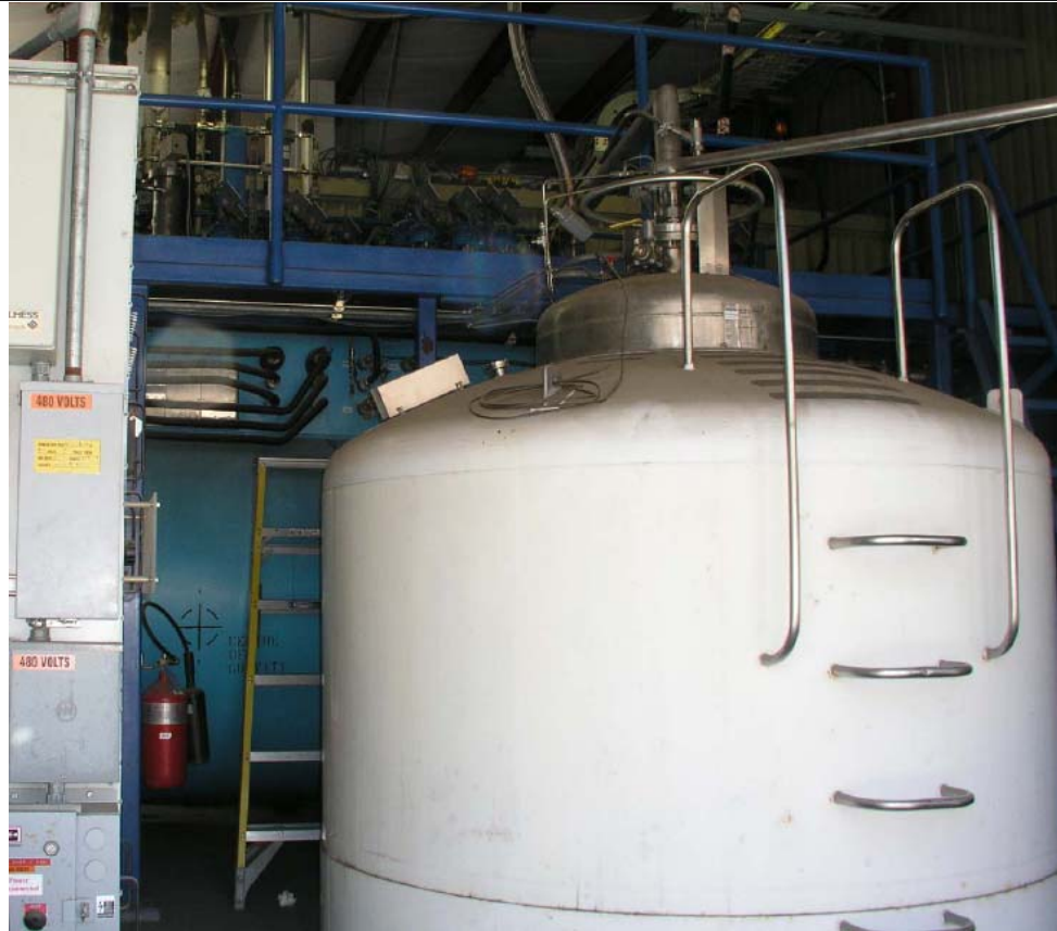
IR2 portion of the cryo plant.
