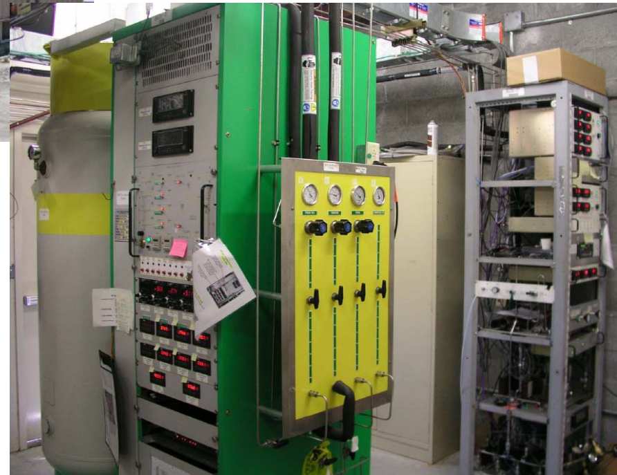
IFR gas mixing racks
