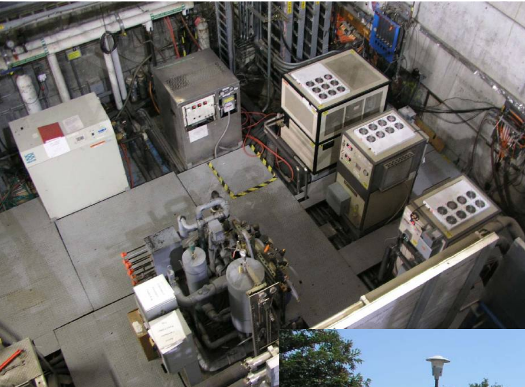
BaBar Chiller Pad
