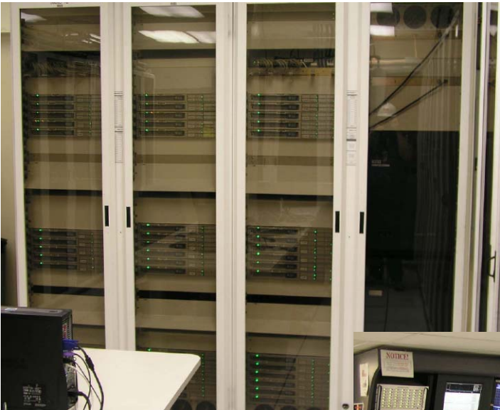
L3 farm & switches
