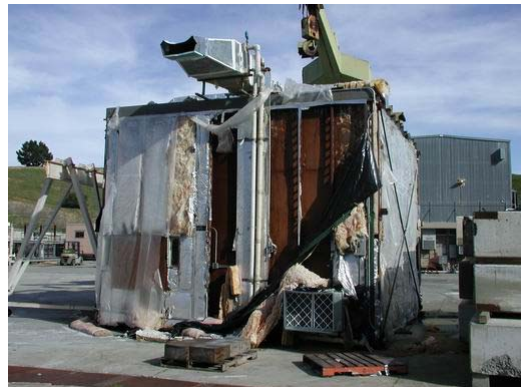
Building 109 "Dry Room"
