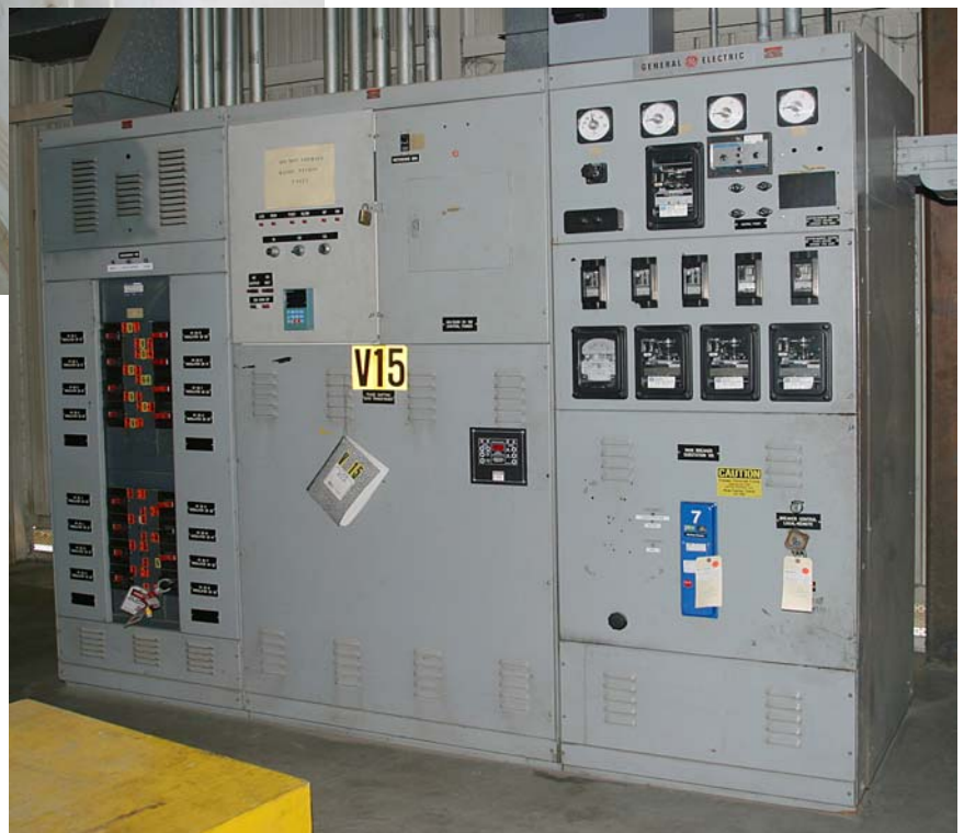
600 V Distribution Section and Controls
