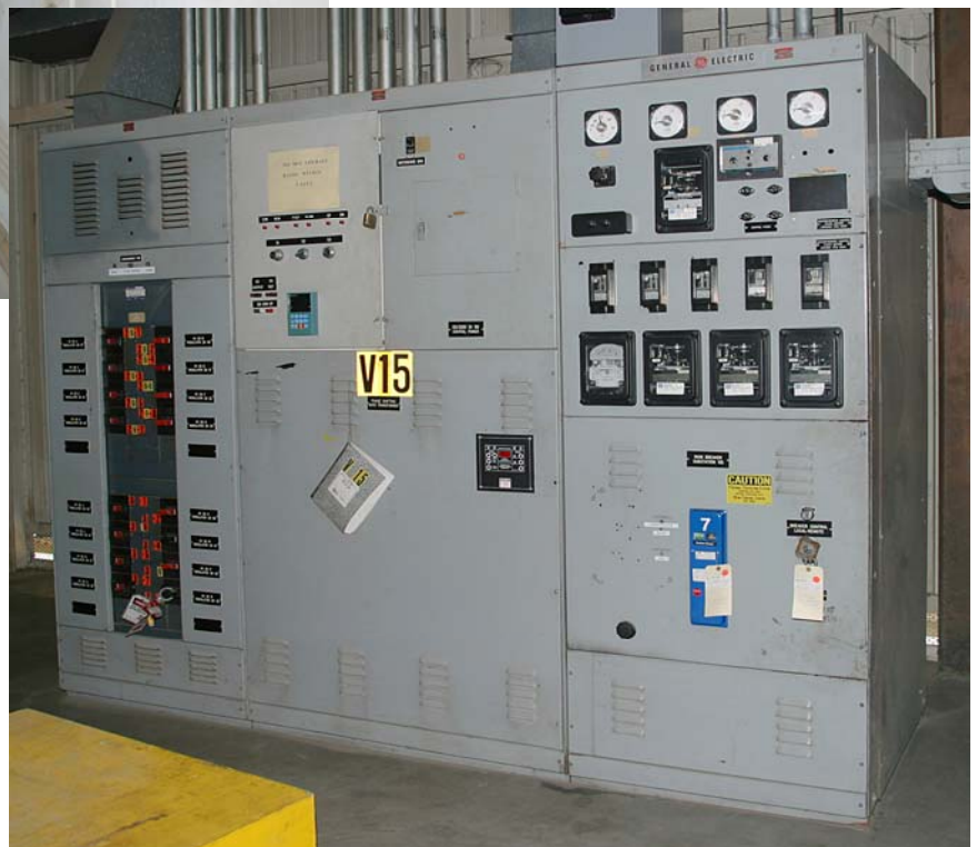
600 V Distribution Section and Controls
