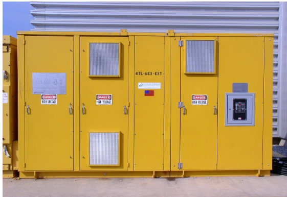
RECTIFIER TRANSFORMER AND FILTERS
