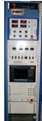
EQUIPMENT CONTROL RACK
